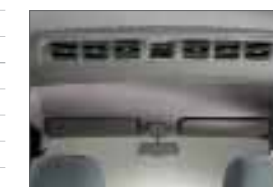
Dual Air Conditioning System
